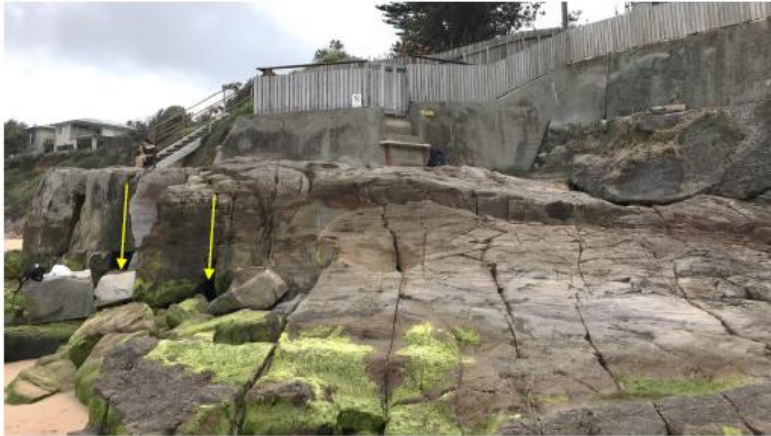
Figure 2-1 Examples of undercut areas (yellow arrows) at subject property (2 January 2018)
